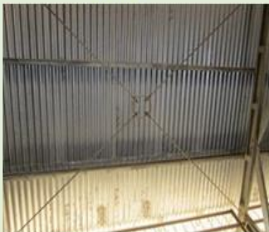
Diagonal Steel bracing to roof
